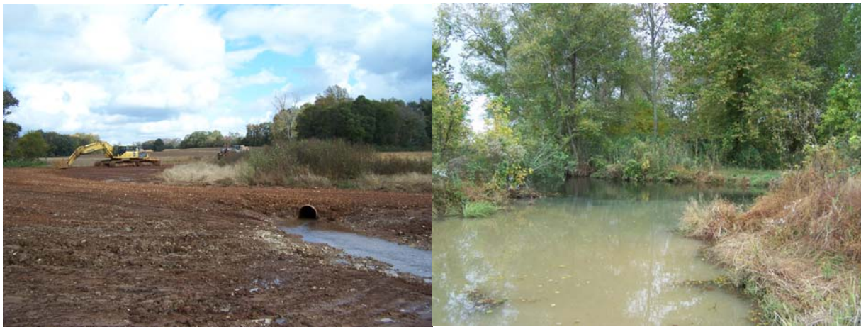
Figure 7. Huntsville sewer line construction, within 50 feet of Beaverdam Creek channel (left) resulting silt load emptying into spring fed ecosystem and E. alabamiae habitat (right)
