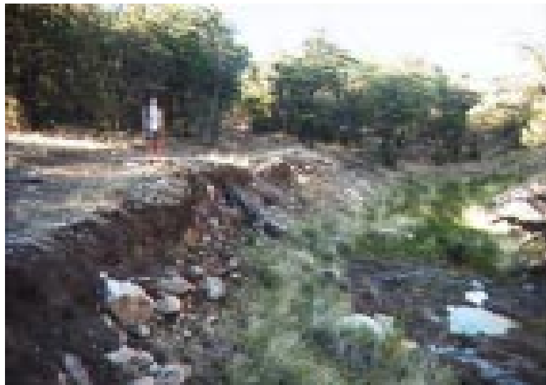
Figure 1 , Road eroding into a stream in the Huachuca Mountains Arizona.
